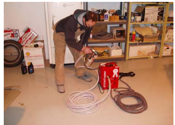
Fig. 1 A Typical HVLP Paint Spraying System includes Dual Compressor with Ventilation Air to the Operator's Face Mask. The Compressor is located outside of the building thereby ensuring only fresh air to the operator.
